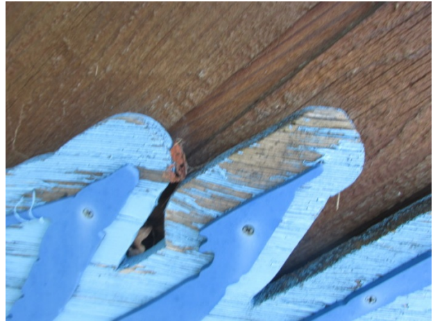
Paint finish deterioration
